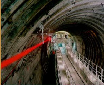
View of the rear of the tunnel boring machine showing the laser guidance system in operation.
